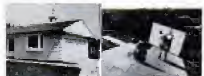
Two-car frame garage amateur can build and getting garage under cover with large sheets of plywood. Both illustrations from the book.
